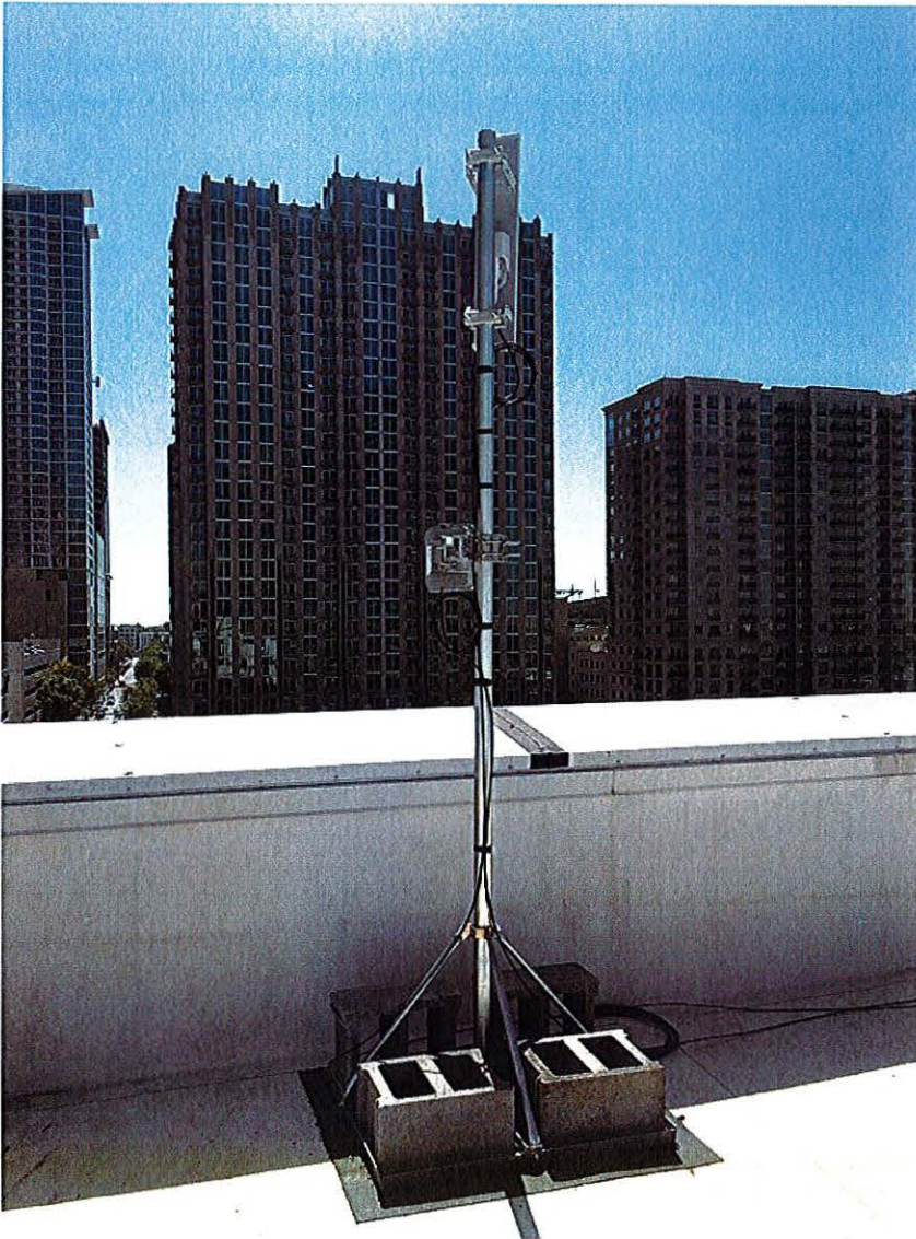
Picture above: Non-penetrating roof mount with mast. This one has a small Wi-Fi sector antenna at the top. The lower antenna is a Type 2 as described above.
