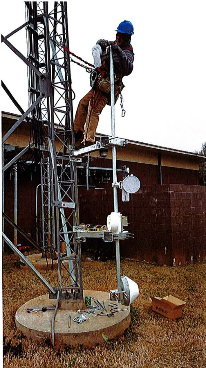
Picture above: Communications Tower attachment – picture taken during preparation before the climb.
