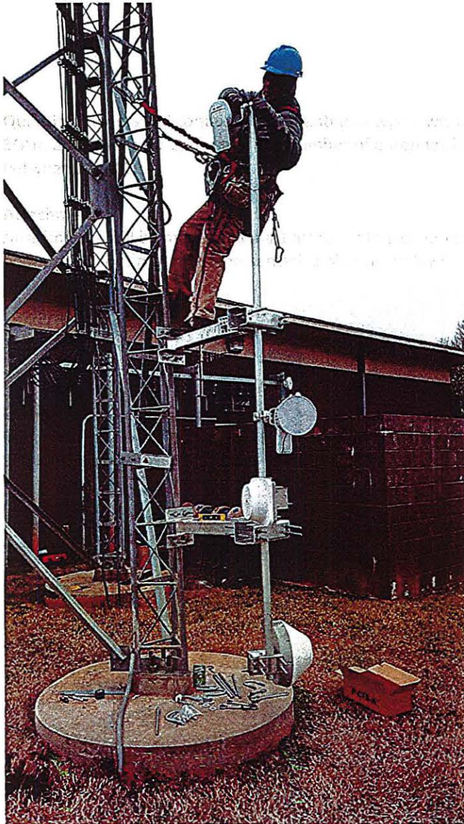
Picture above: Communications Tower attachment – picture taken during preparation before the climb.
