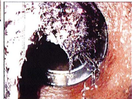
Roots at Service Lateral Connection
