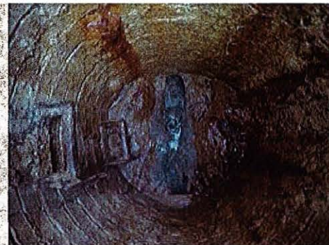
Manhole w/ active infiltration (stains)
