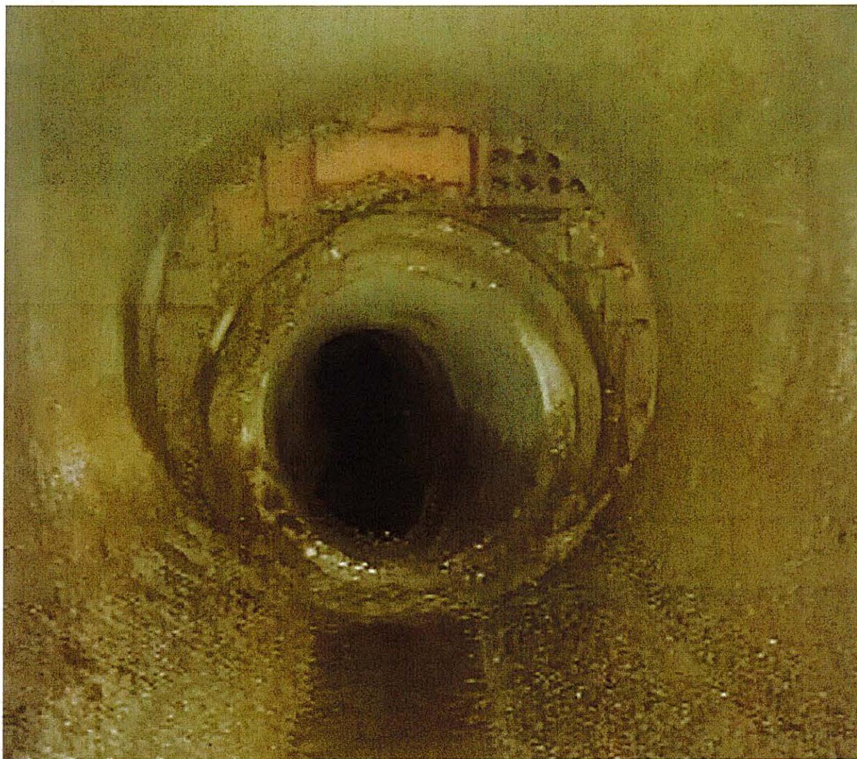
Wayne County Executive Jetport, Screen Shot from CCTV Video - Ditch to Drop Inlet (2025-07-25) of 24" RCP at connection to 18" RCP.
