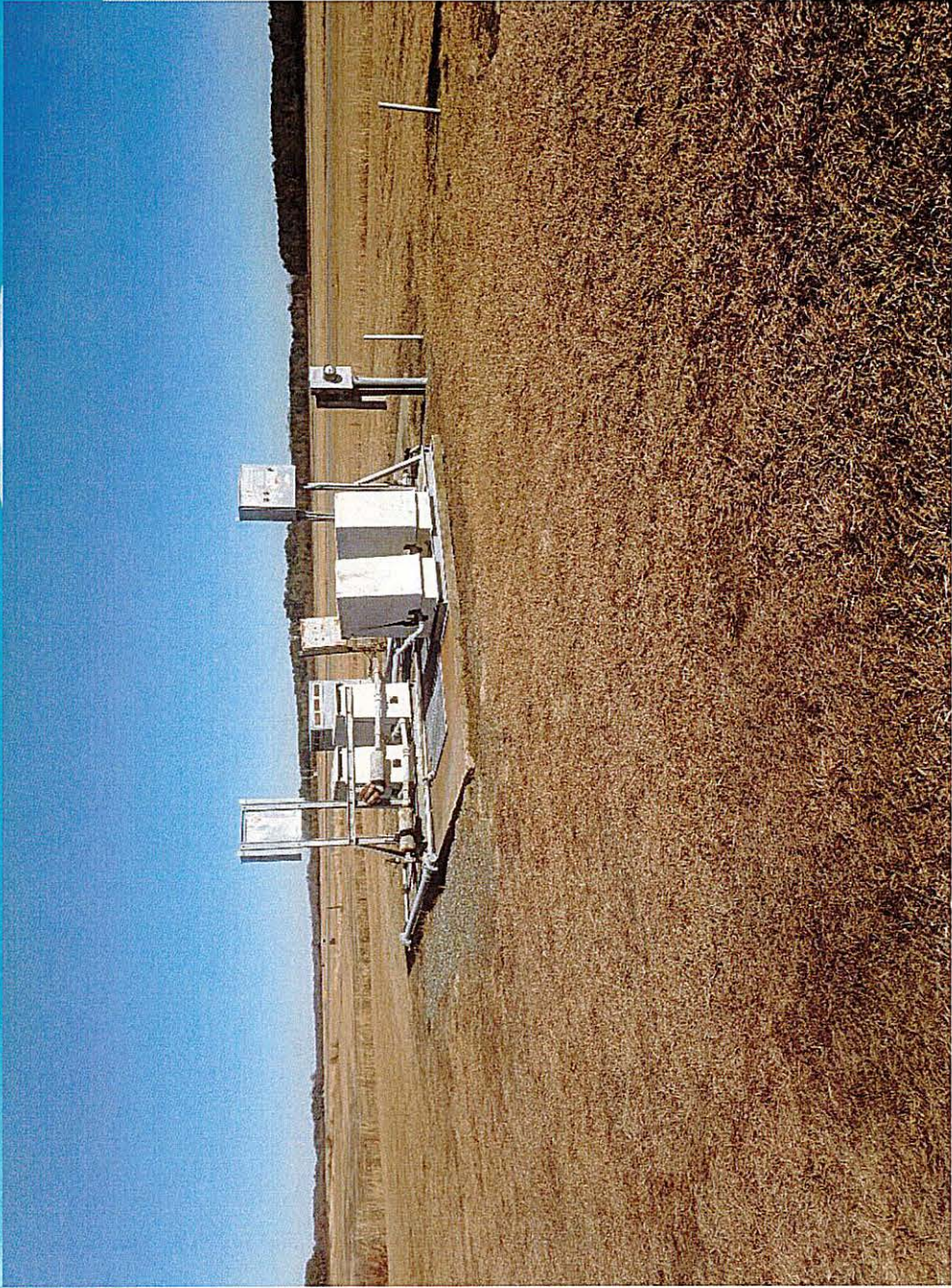
Aging Lift Station
